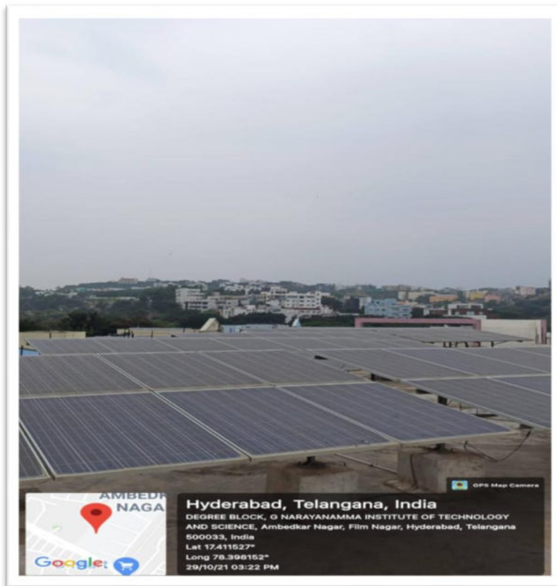
7.1.2.1. Solar Energy – Solar Panels at F – Block Terrace
