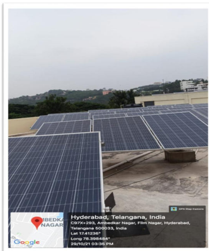
7.1.2.1. Solar Energy – Solar Panels at CSE – Block Terrace
