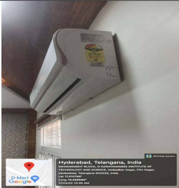
7.1.2.5. Use of ACs / Power Efficient Equipment at ECE Block
