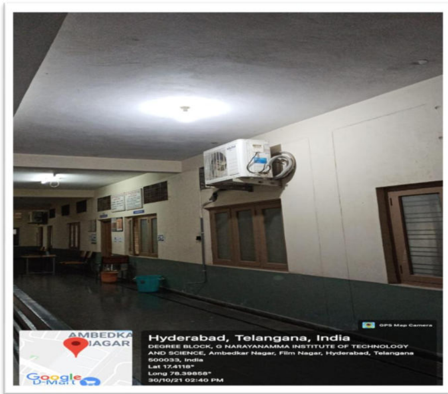
7.1.2.5. Use of LED Bulbs / Power Efficient Equipment at F- Block
