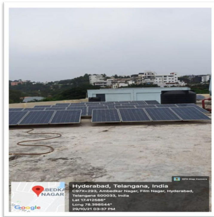
7.1.2.1. Solar Energy – Solar Panels at ECE – Block
