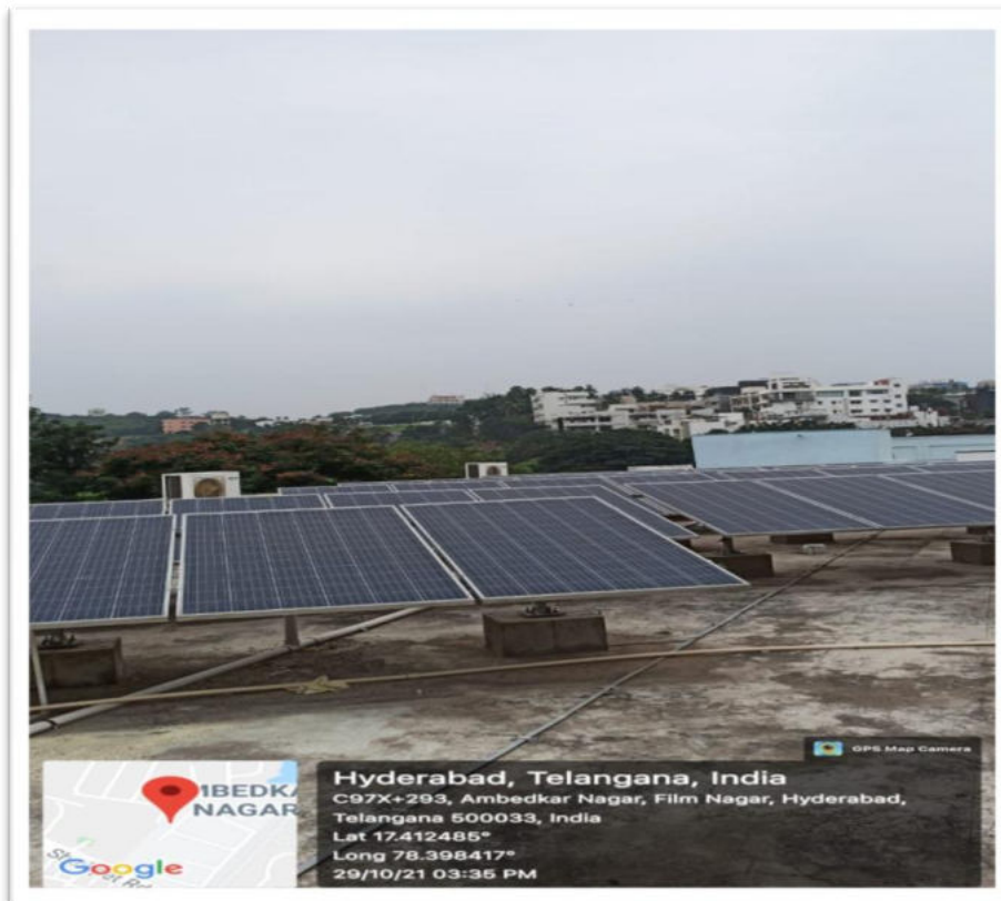
7.1.2.1. Solar Energy – Solar Panels at ECE– Block Terrace
