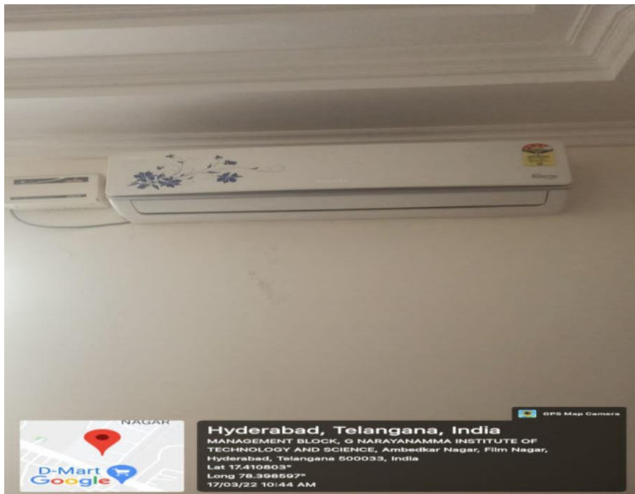
7.1.2.5. Use of ACs / Power Efficient Equipment at EEE Block
