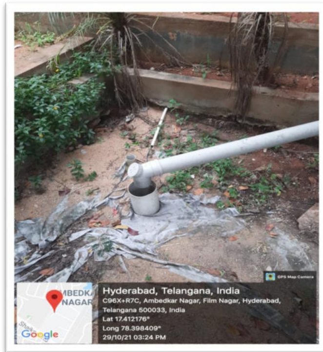
7.1.4.2. Bore Well / Open Well Recharge at EEE Block
